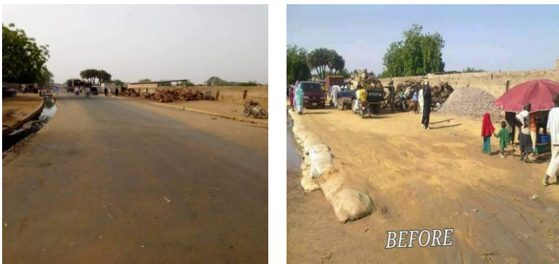
Figure 9. Newly Constructed Gawon Dogari Hadejia Township Road Old Gawon Dori Hadejia Township Road 2015.
